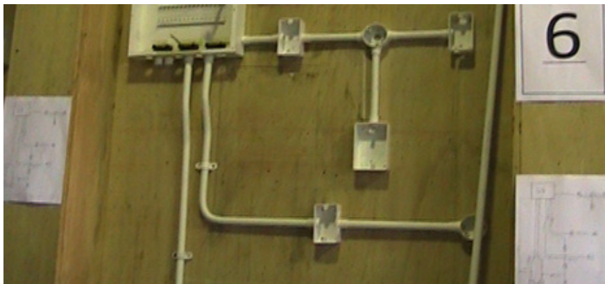
Figure 18: A partially completed task, showing one student's work-station number, diagram of wire-way, and the student's work
